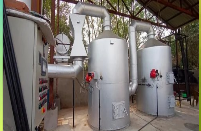
BIO MEDICAL WASTE INCINERATOR
