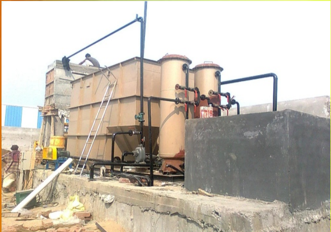
S.A.F.F Sewage Treatment Plat
