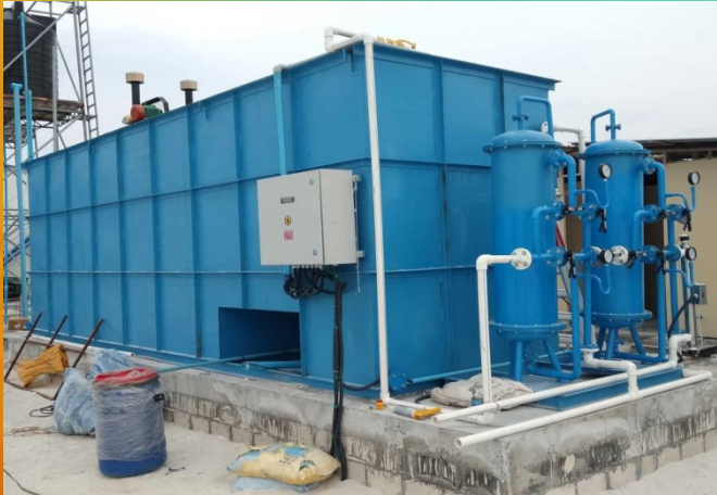
M.B.B.R Sewage Treatment Plant
